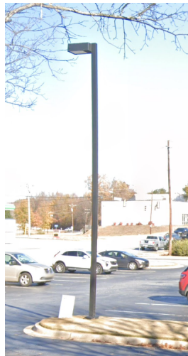
Figure 8: Sample Parking Area Lighting
